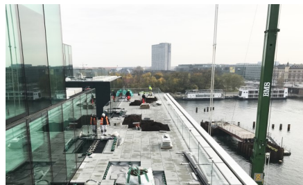
The planting beds were equipped with System Build-up "Roof Garden" with Floradrain® FD 40-E.
